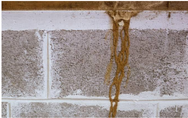
Figure 15 Subterranean Termites, Cement/Masonry
