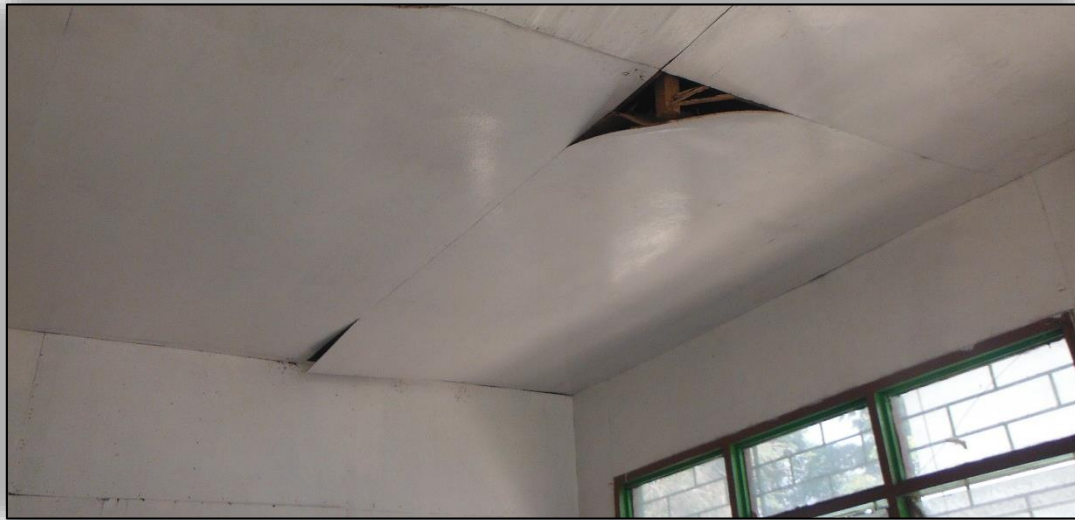
Figure 4 Sagged Plywood Ceiling
