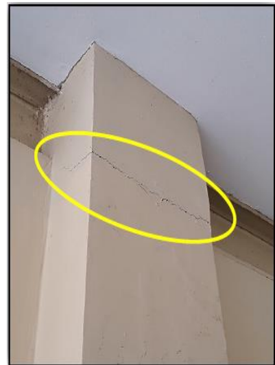
Figure 6 Crack on Column
