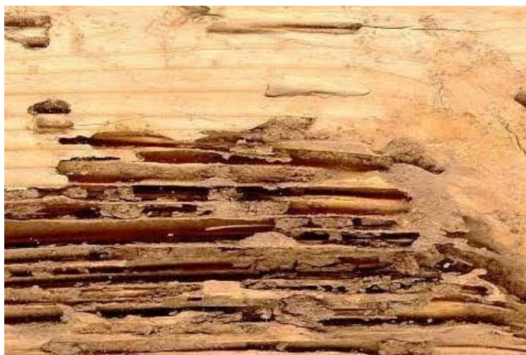
Figure 16 Subterranean Termites Wood Damage
