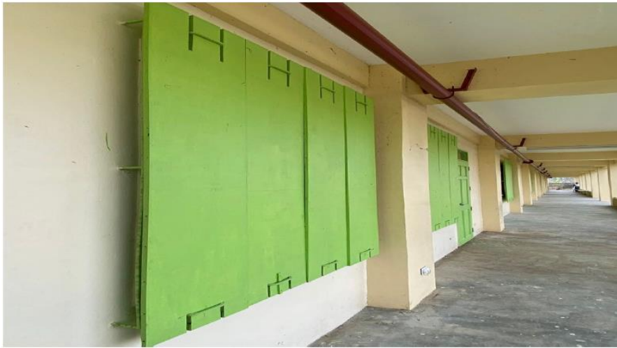
Figure 12 Proposed replacement to Window shutters: To get Material needed, Installation Procedure and Corrective measures to implementing SDO
